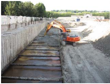
Extraction under the water table: sheet pile section and shoring up with piles
