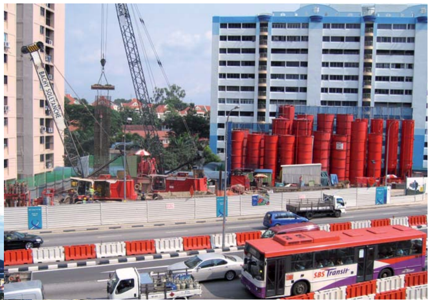
General view of the bentonite plant and the construction of the retaining walls for a station entrance
