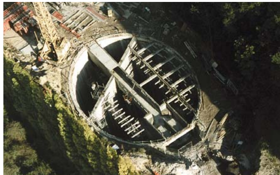
FRANCE - Méricourt Integrated shaft for deep storm tank - 1 st innovation prize FNTF
