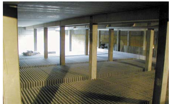
FRANCE - Lons le Saulnier Montmorot settling tank
