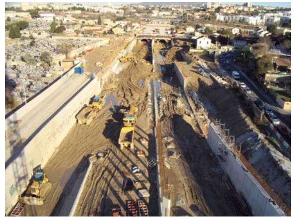
FRANCE - Marseille La Parette cut and cover
