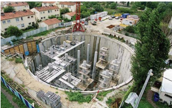
FRANCE - Bordeaux - Floirac Storage tank Alfred Giret
