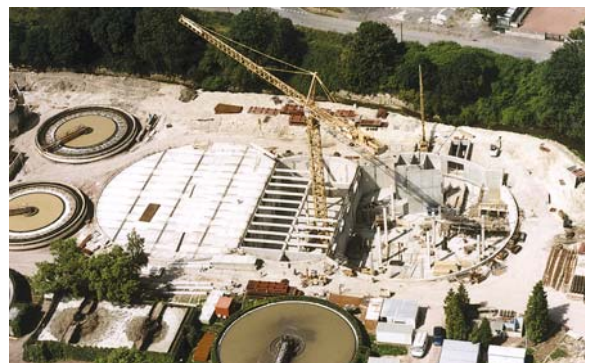
FRANCE - Arras Storage tank for the treatment plant
