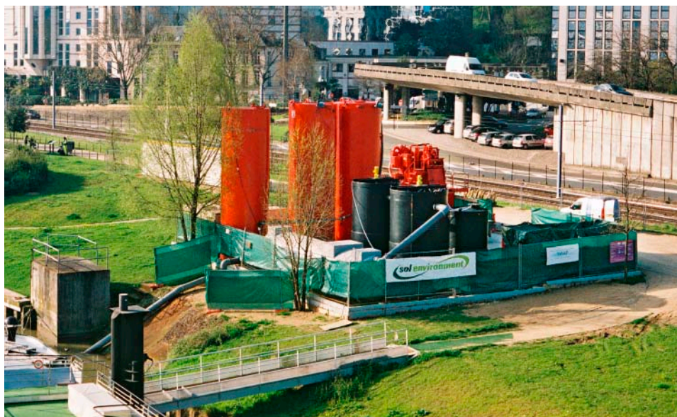
Temporary treatment plant
