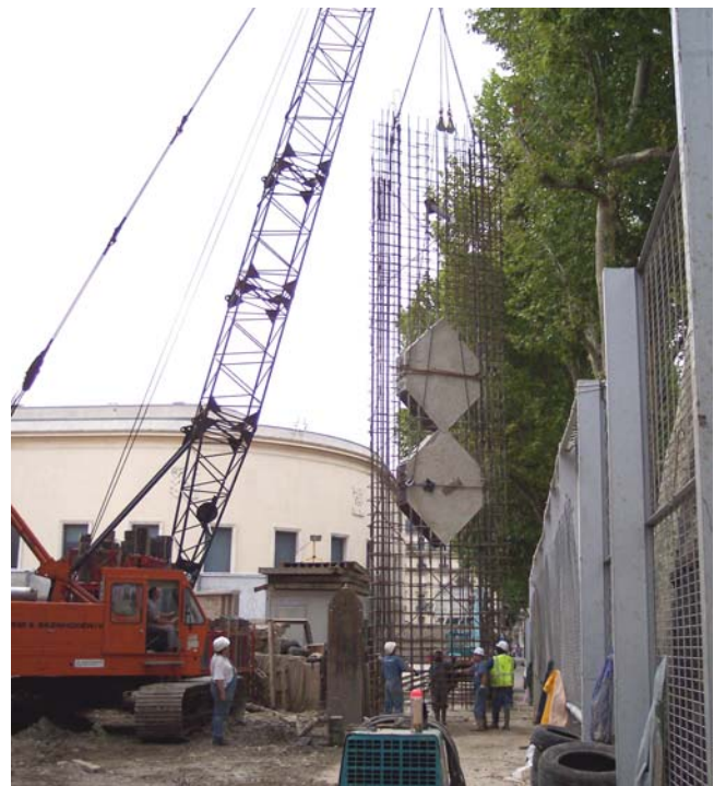
The tunnel boring machine's route for the construction of water supply pipes from the pumping tank called for the installation of boxed out sections consisting of metal boxes filled with cement slurry in the diaphragm wall reinforcement cages
