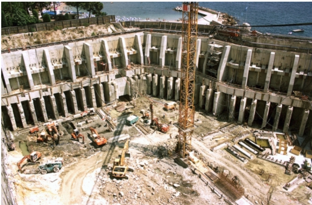
View of the north part of the site and of the ground support (rib of the T walls, load transfer slab, buttresses)
