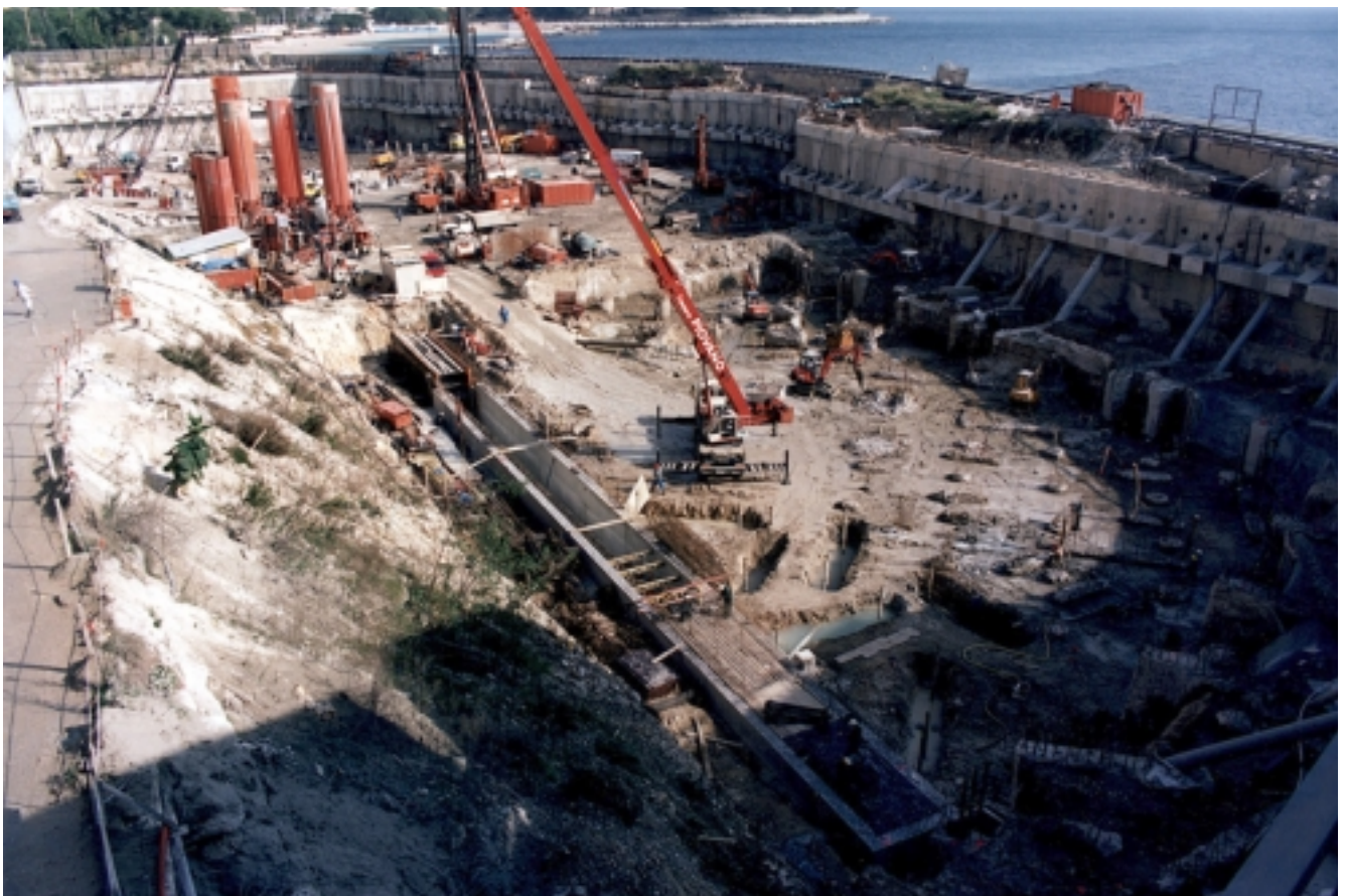
Plan view of the southern part (drainage tunnel, excavated foundations, small struts installed)
