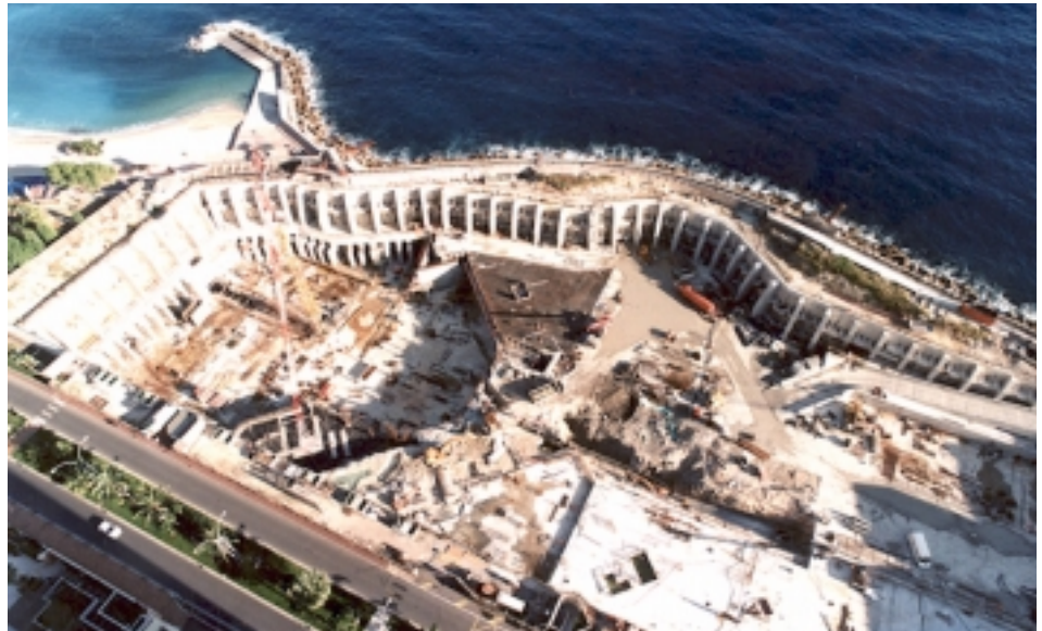
Overall view of the site (diaphragm wall with buttresses, T walls, slabs)
