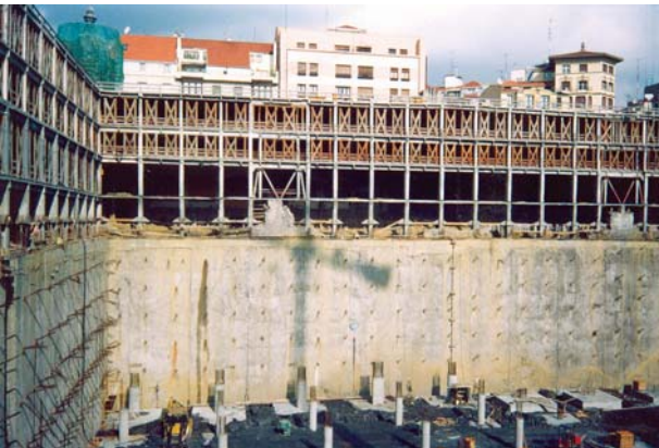
Example of a diaphragm wall supported by 5 levels of ground anchors used for constructing basements as part of a refurbishment project undertaken inside an historic building where only the facades were retained.
