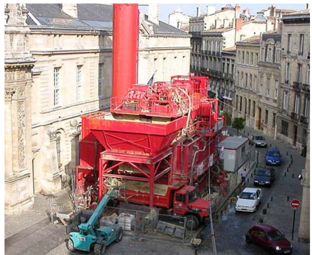
Drilling slurry production and processing plant comprising mixers, pumps, vibrating screens, centrifuges, bentonite powder storage silos, new and spent slurry storage silos.
