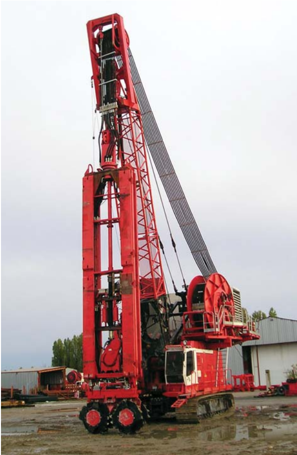
Hydrofraise mounted on its crane. The spoil is dislodged by the rotating drum cutters and pumped to the surface with the drilling slurry. The drilling slurry is used to stabilise the excavation and to facilitate the transportation of the spoil to the surface. The drilling tool descends in a continuous operation as it excavates the trench.
