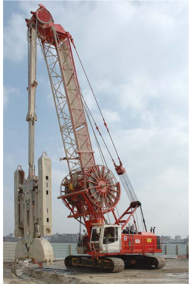
The KS2 hydraulic grab. The spoil contained in the grab buckets as they close is removed to the surface by the grab. Drilling slurry is only used to stabilize the trench. Excavation proceeds sequentially during which the grab is alternately raised and lowered.
