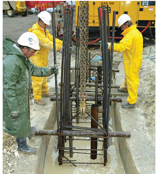
Positioning and setting a reinforcement cage on guide walls. Reservation tubes attached to the cage are clearly visible and can be used for non-destructive testing of the concrete, to carry out drilling and grout injection at the base of the wall.
