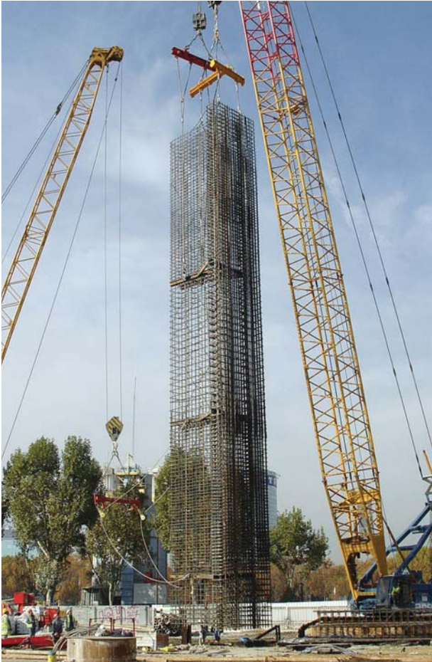
The installation of a reinforcement cage using a service crane. Special case of a reinforcement cage for a 'T' shaped panel section.
