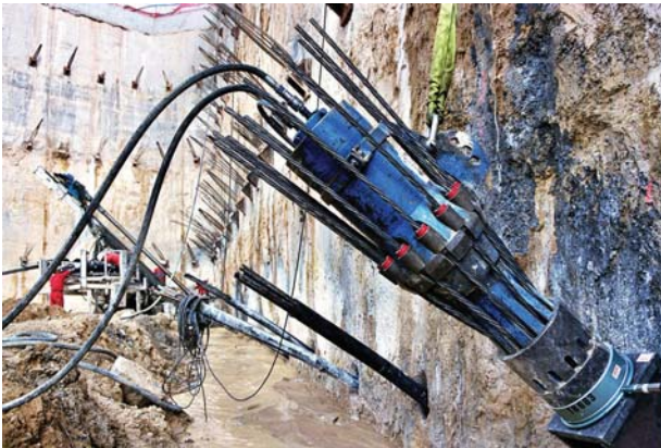
Ground anchors can consist of single bars or a number of strands. They are pre-stressed using a hydraulic jack. The photo shows a strand anchor as it is being pre-stressed.
