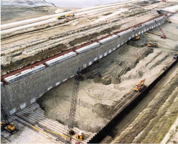
Case of passive ground anchor blocks positioned at the back of a quay diaphragm wall. They are anchored at the other end to a sheet pile wall.
