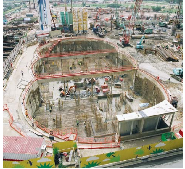
Multi-cell wall with self-stabilising circular segments with props at the intersections only.
