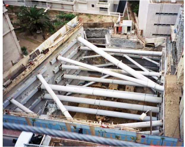
Support wholly provided by props. As in the case of passive anchors, the props will only take load if the wall moves.
