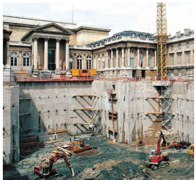
Example of a deep trench adjacent to a historic building, below the water table level, protected by a wall combining pre-stressed ground anchors and corner struts.
