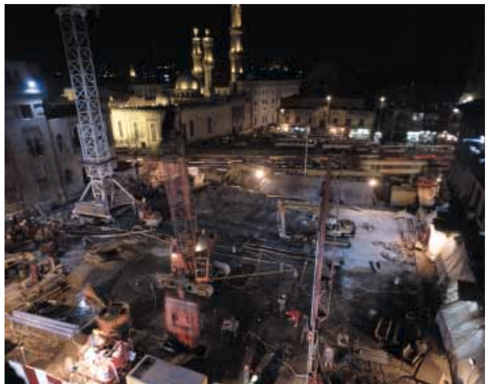
El Hussein ventilation station
