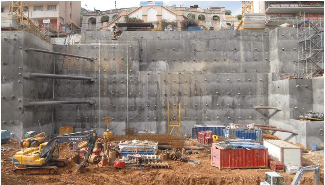
Several layers of prestressed anchors and angled struts were used for temporary support for the Berlin wall
