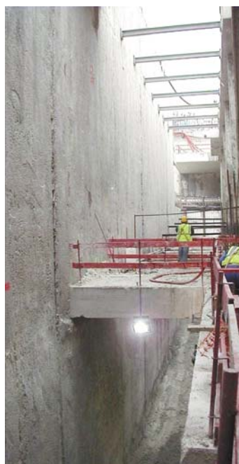
Excavation floor at a depth of 32 m and a 27 m head of water
