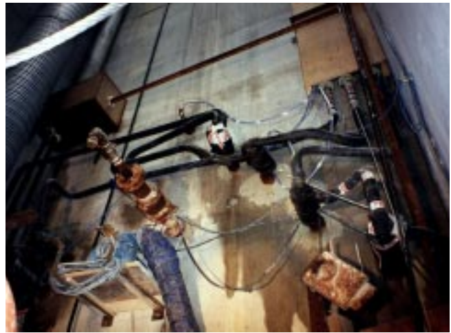
Liquid nitrogen pipe
