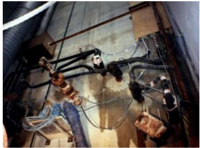
Liquid nitrogen pipe
