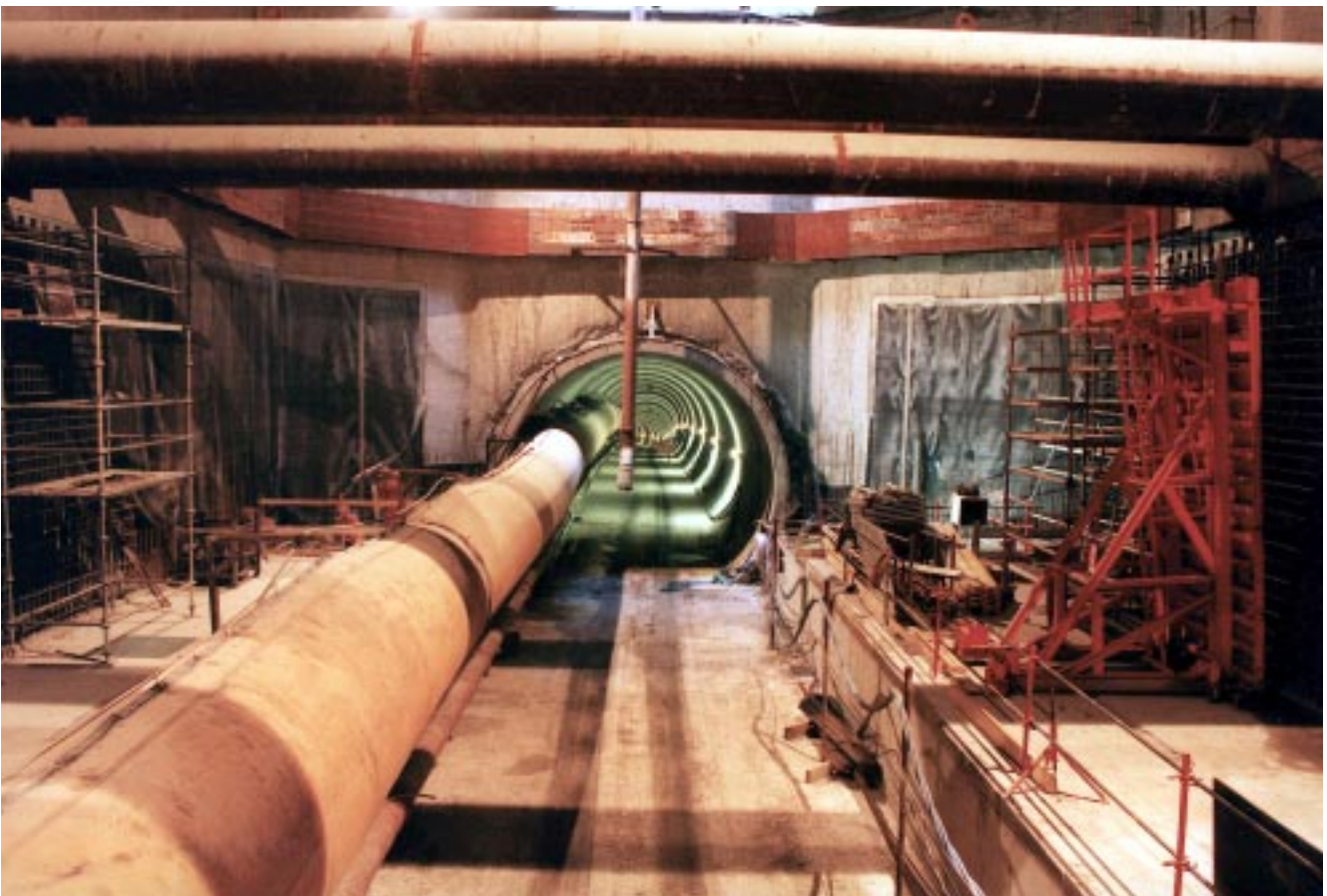
Crossing Pavé de Lille station
