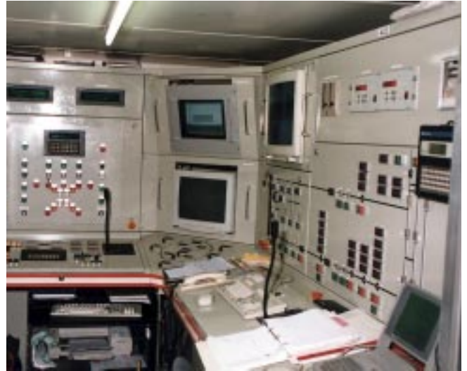
TBM operator's position
