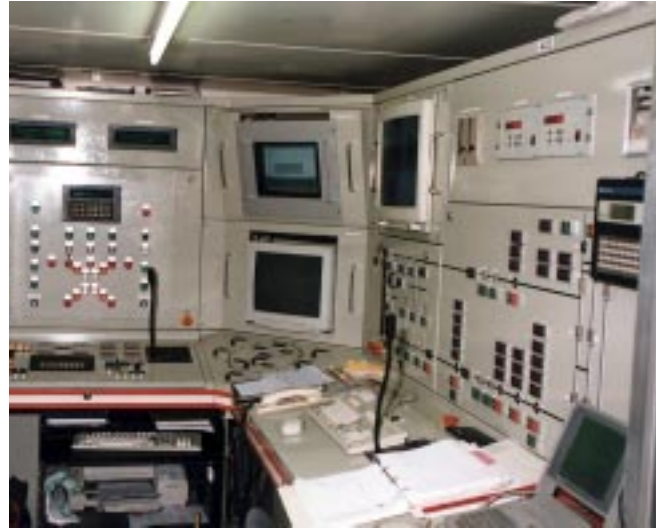
TBM operator's position
