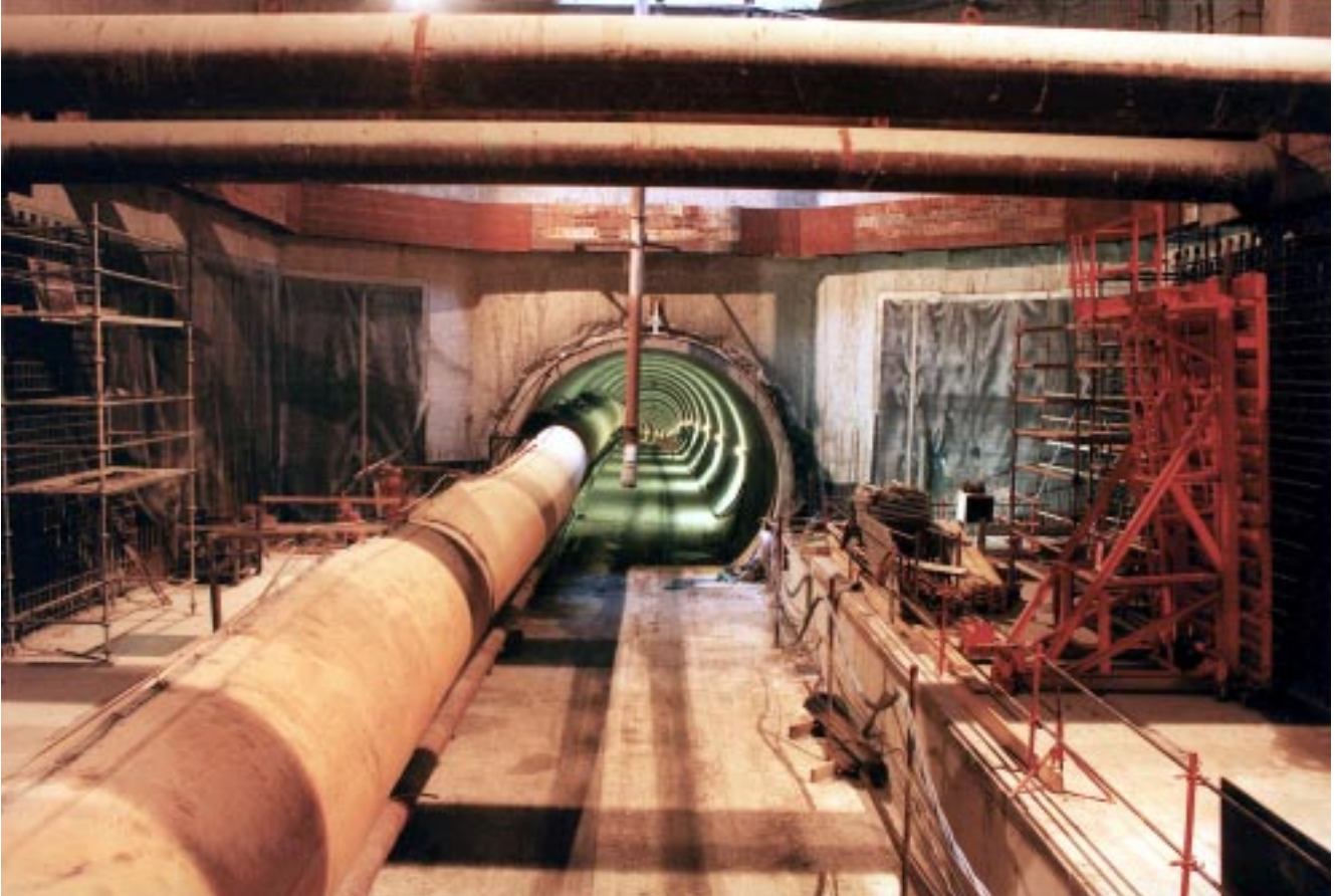
Crossing Pavé de Lille station
