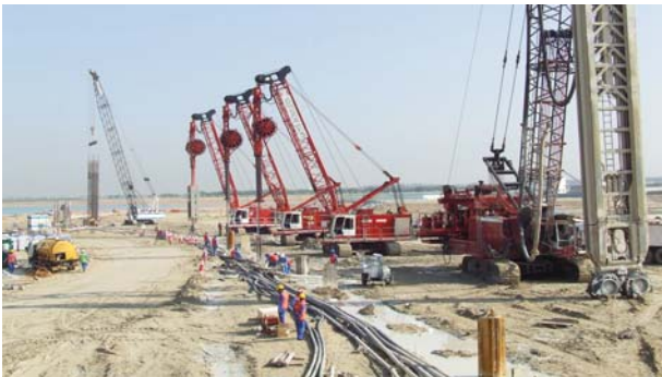
UNITED ARAB EMIRATES - Abu Dhabi - Al Raha Beach Diaphragm wall for a 12km long quay wall
