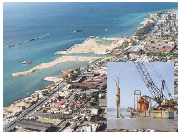
GREECE - Port of Patras Construction of a 1,000m pier and a 500m quay
