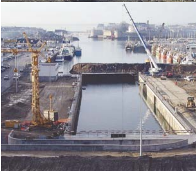
FRANCE - Concarneau Dry Dock
