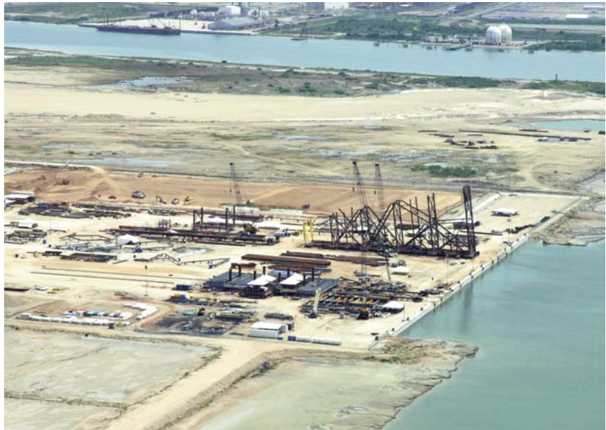
View of the terminal in October 2008. Platforms being fabricated are visible on the two Correderas.
