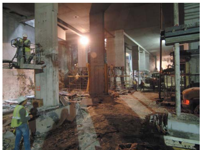
Excavated bottom at 5.20 NGM, peripheral sawing and sprayed concrete shell, RC sealing of down columns as work progresses
