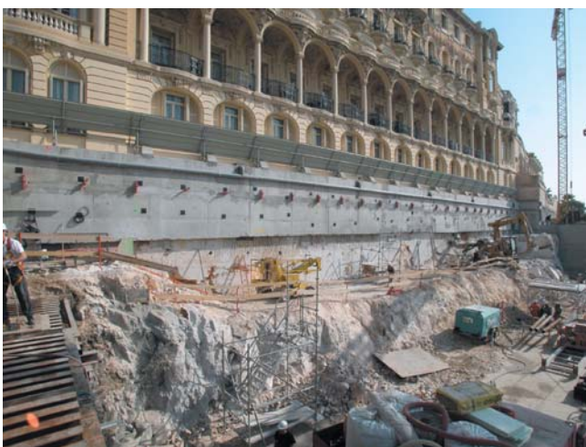
Reinforcement by anchorages under the Hotel and the first concreting work of the support wall
