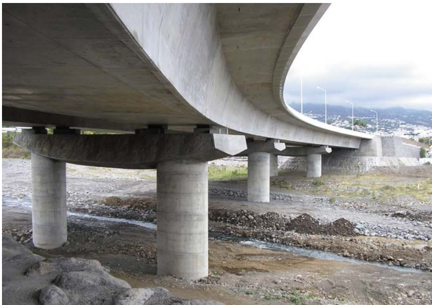
View of the completed structure from the abutment on the right bank
