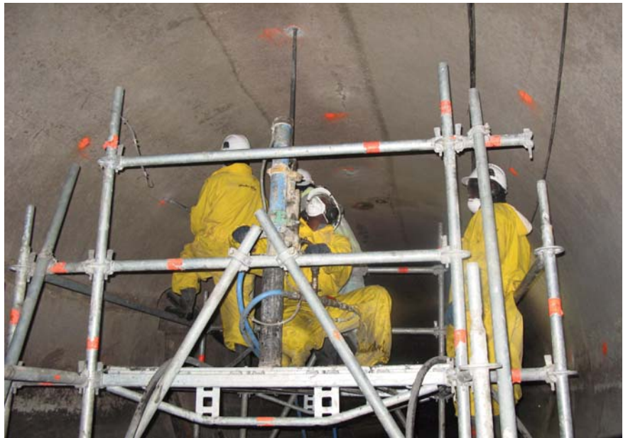
The effluent channel is a confined space which meant additional protective material had to be worn, such as gas detectors and safety headphones to protect against the noise accentuation.
