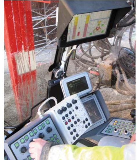
The rotating drums carry out the boring and mixing of the soil and cement.
