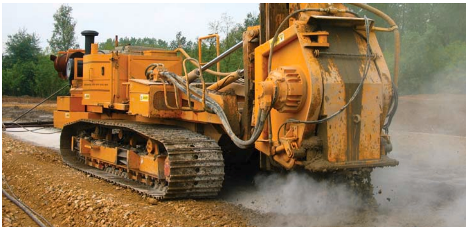
Installation of 21 000 m 2 of Trenchmix® for settlement control underneath a storage area.
