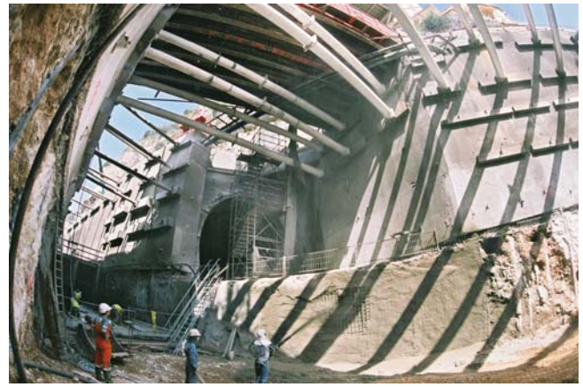
The upstream head, intersection between the service tunnel and the T33 tunnel
