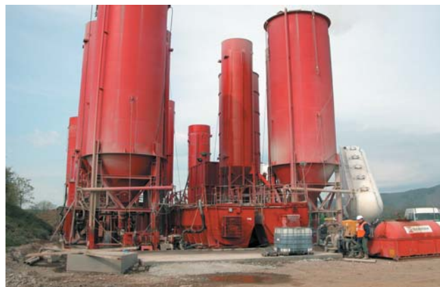
Slurry plant (50 m 3 /h)
