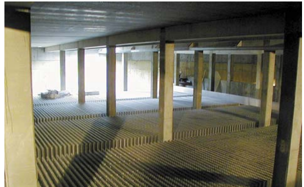
FRANCE - Lons le Saulnier Montmorot settling tank
