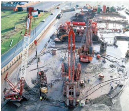
UNITED KINGDOM - Blackpool Storage tank
