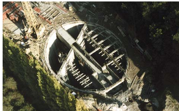
FRANCE - Méricourt Integrated shaft for deep storm tank - 1 st innovation prize FNTF
