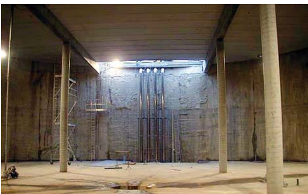
FRANCE - Anglet Pechmeja storm tank
